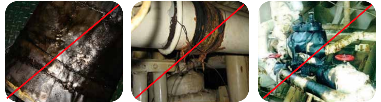
Oily lagging in fuel piping, sea water pipe patched
