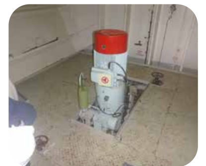
Emergency Fire Pump
